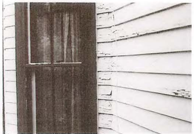
Fig. 8 Peeling to bare wood—one of the most common types of paint failure—is usually caused by an interior or exterior moisture problem. Photo: Anne E. Grimmer.
