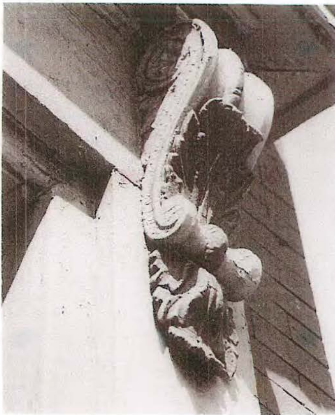
Fig. 1 Excessive paint build-up on architectural details such as this ornamental bracket does not in itself justify total paint removal. If paint is cracked and peeling down to bare wood, however, it should be removed using the gentlest means possible. Photo: David W. Look, AIA.
