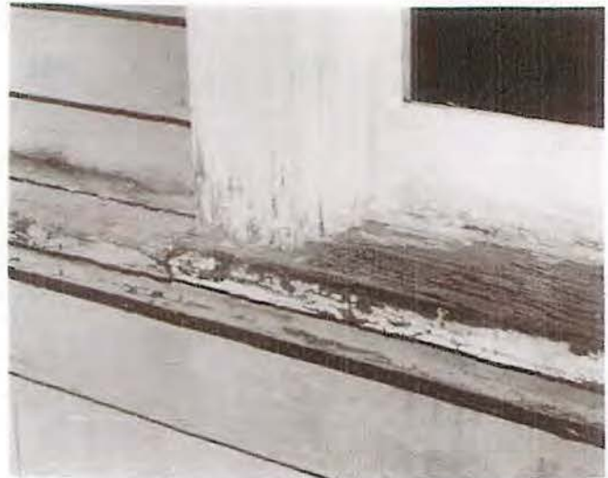
Fig. 4 Paint films wear unevenly depending on exposure and location. Exterior locations which are susceptible to accelerated deterioration are horizontal surfaces such as window sills. These and similar areas will require repainting more often than less vulnerable surfaces. In the case of this window sill where paint has peeled off and adjacent areas have cracked and alligatored, the paint should be totally removed. Prior to repainting, any weathered wood should be rejuvenated using a solution of 3 cups exterior varnish, 1 oz. paraffin wax, and mineral spirits/paint thinner/or turpentine to make 1 gallon. Liberal brush application should be made. This formula was tested over a 20-year period by the U.S. Department of Agriculture's Forest Products Laboratory and proved to be just as effective as water-repellent preservatives containing pentachlorophenol. After the surface has thoroughly dried (2-3 days of warm weather), the treated surface can be painted. A high quality oil-base primer followed by two top coats of a semi-gloss oil-enamel or latex-enamel paint is recommended. Photo: Baird M. Smith, AIA.
