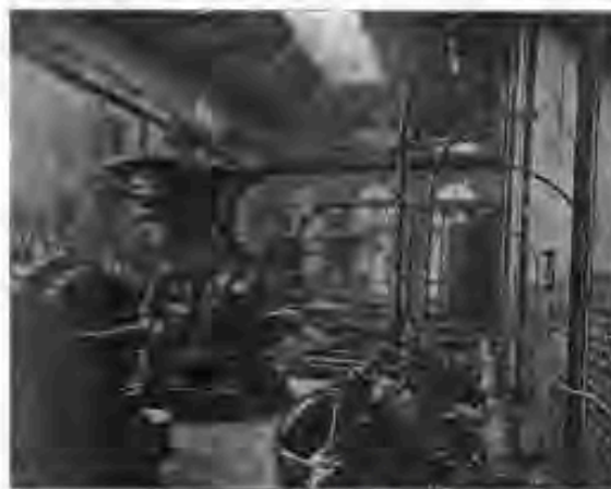
Three Main Units in Turbine Room.
