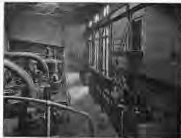
Exhaust and Swirlworks in Turbine Room.
