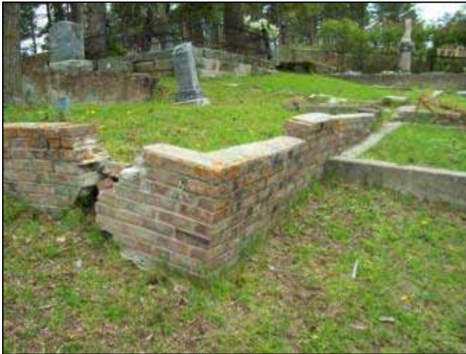
Figure 3.8 – Uneven settlement of brick wall with mortar
