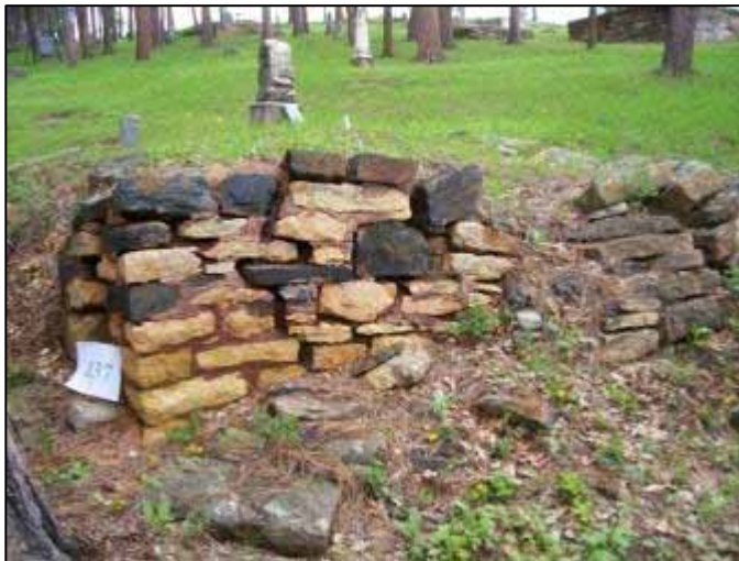
Figure 3.9 – Uneven Settlement of Stone Wall with Mortar
