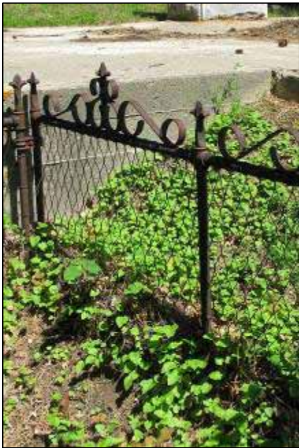
Plant litter and soil building up along plot fence is a factor in deterioration of the bottom portion of this ornamental iron fence.
